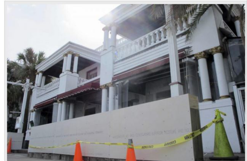
FILE PHOTO In this Oct. 28, 2016 photo, one of the many businesses on the St. Augustine waterfront is being repaired after it was damaged by flooding during Hurricane Matthew. More than 1,000 historic homes and buildings were damaged by storm surge, a University of Florida team has found. Water flooded all seven of St. Augustine's federally designated historic districts last month. (AP Photo/Jason H. Dearen)
